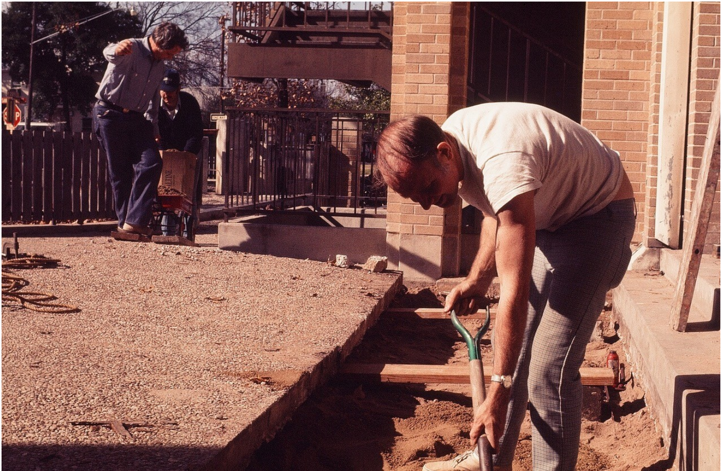
2/76 John Camden and John Towery (pastor of the church from 1959-1989) bringing more sand to Mel to help level the courtyard
