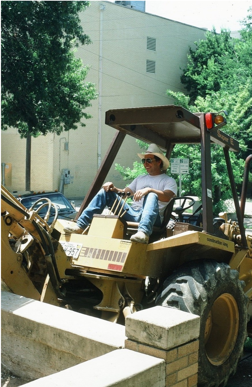
1987 A relaxed Danny Masters (son-in-law of John Towery) using heavy equipment to break up the courtyard and take down the stone blocks in the playground.
